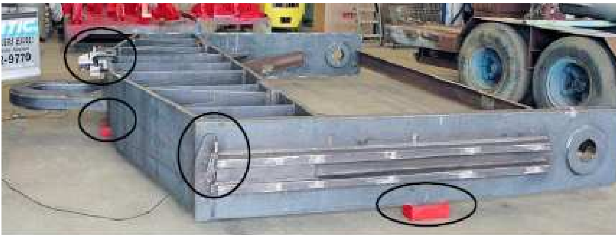
Figure 1: VSR SETUP. The vibrator (circled) was placed above the lifting lug, and clamped using the front flange of the BL-8 Vibrator. The BL-8 Vibrator has two sets of mounting flanges, which allows effective orientation of the Vibrator relative to the work-piece.
